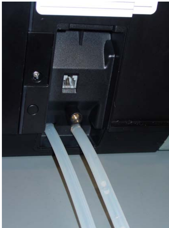
Drain Tubes with Access Panel removed
